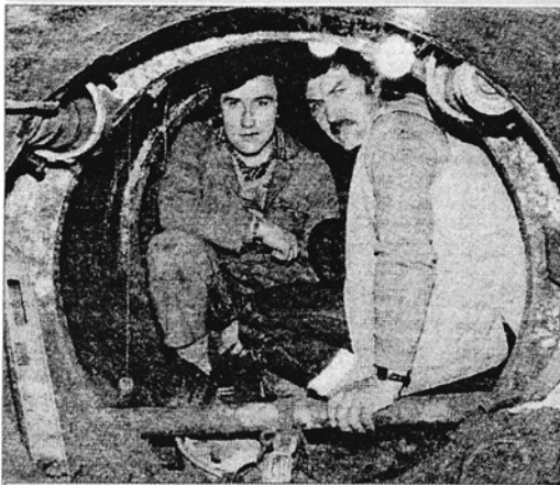
Gerald Davey (left) and Malcolm Adnett five metres down, in Dereham's new sewerage system.
