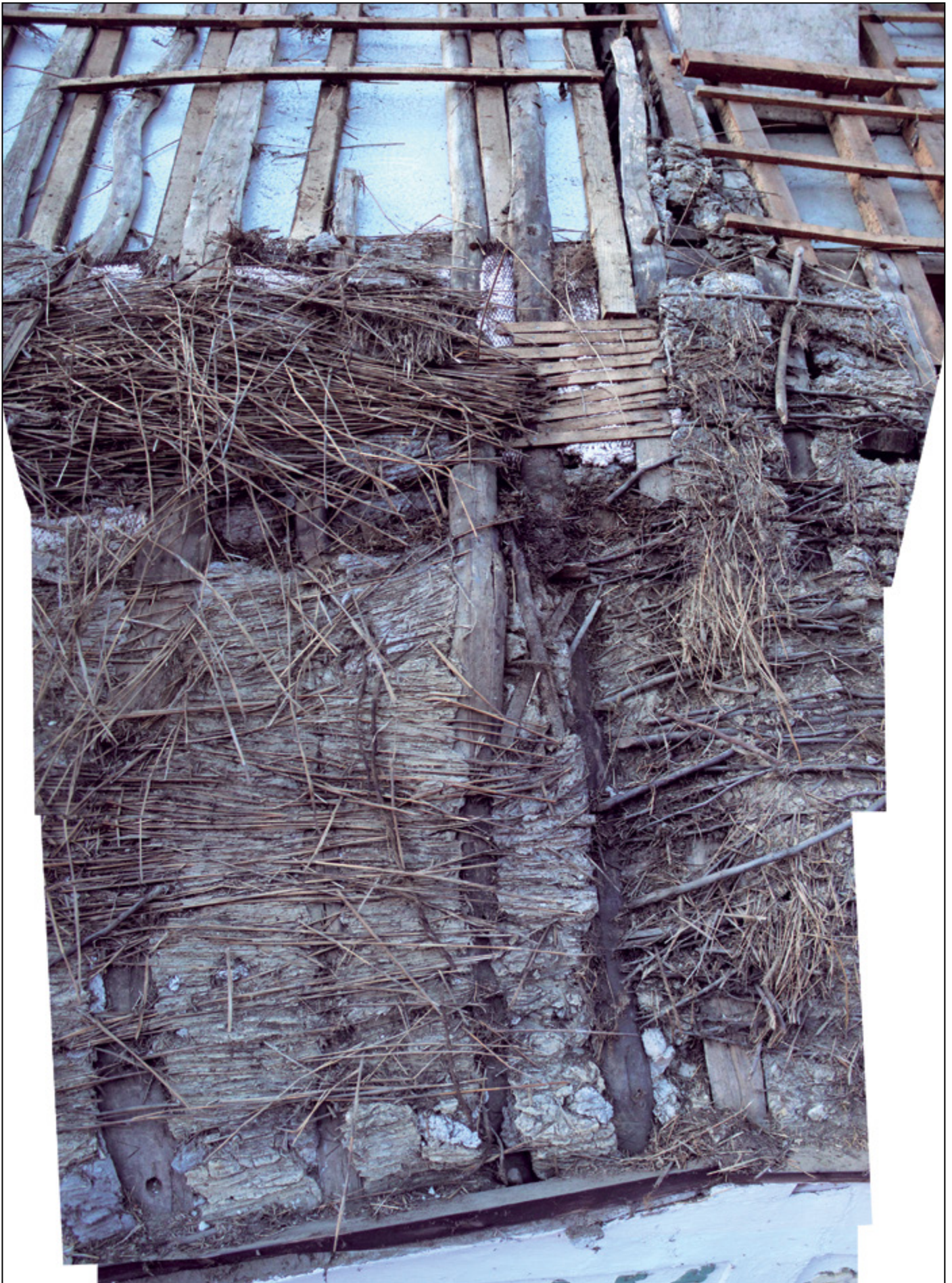
East face of roof, section north of pitched dormer window. The vertical rafters from left to right are the run of four with carpenters marks at base. The first timber is VIII the 2nd has the arrow mark representing 9, then X and XI. The building alignment changes after timber XI and the method of thatching changes at the same point, indicating a different phase in the building's development. The base layer of thatch on the left, running horizontally, is water reed, this is the only surviving area where reed was found embedded in daub; however here the daub was applied from the outside. No split (riven) wood laths or nails were used in this section of the roof.
