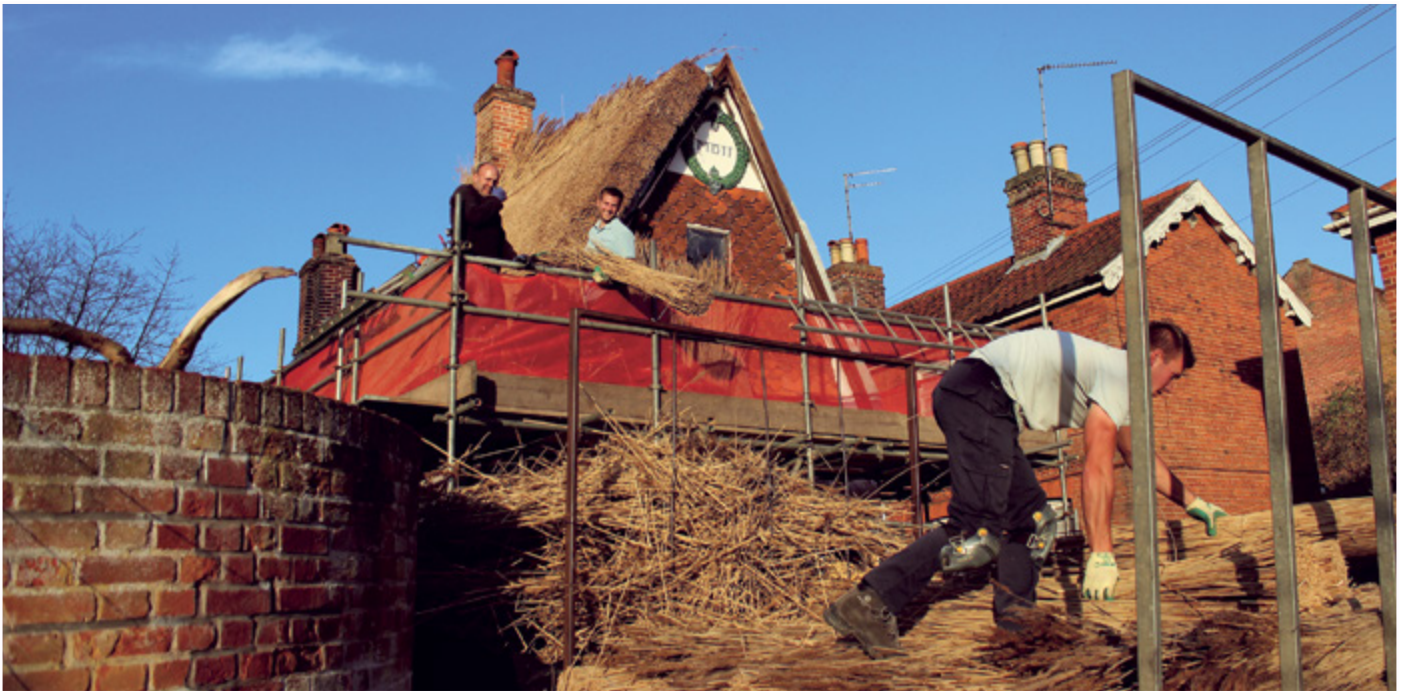
M & B Thompson Thatchers at work on the roof of the museum on 28th October, The craftsmen from left to right Marcus Thompson, Tom Lloyd and Miles Gray.
