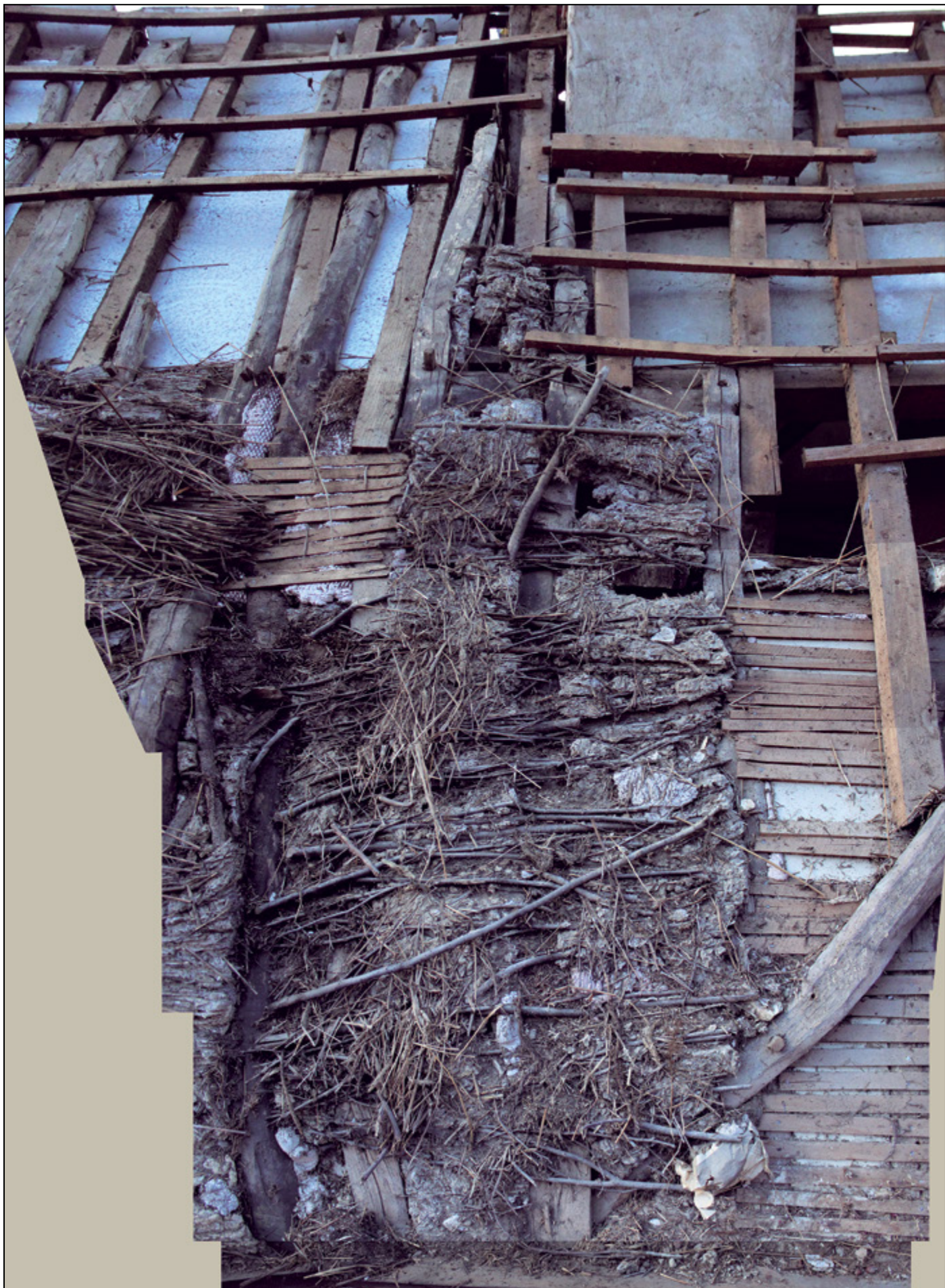
East face of roof, South of the central dormer window (overlaps with photo on previous page). The vertical timber on the left is timber XI. The two sections of horizontal timber wall plate (bottom of photo) butt together at the point the building alignment changes. The thatch on this section of the roof is Rye straw on hazel rods and daub base.
