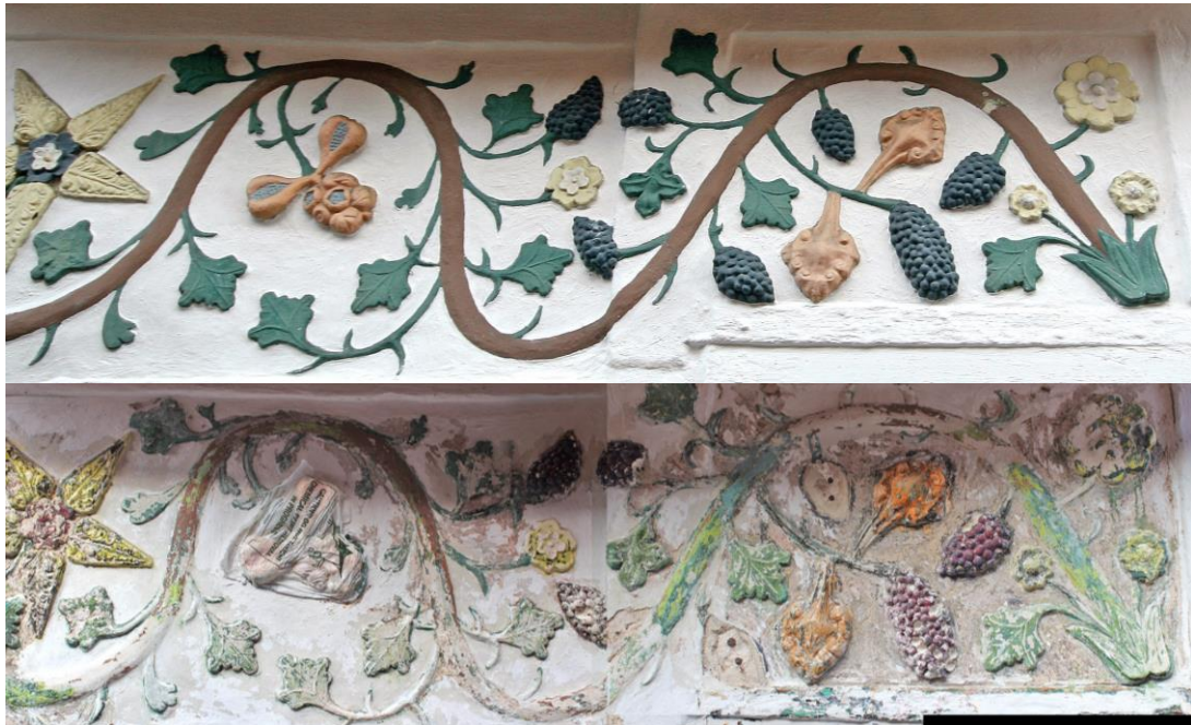
A section of the pargeting before and after the the vigorous work on the paint. The missing bunches of grapes to the right of centre are now stored. The tops of the steel pins to which they were fixed can be seen. The plaster will now have to be protected for the winter, and restored in the spring.
